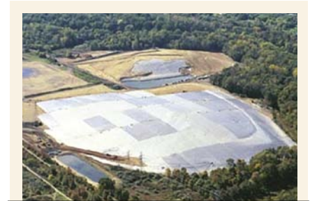
Photo 6. Two cells at Crown Vantage Landfill were lined with PVC geomembrane. The seams were air-channel tested using the procedure described in this article.
