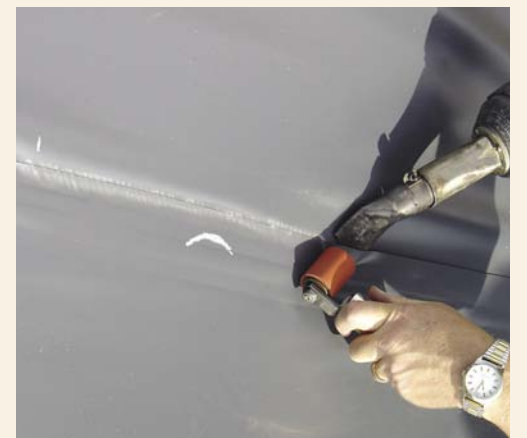
Photo 5. Hot air welding the upper flap of the geomembrane six inches above and below (see small tic mark near arrow) an aneurysm (large mark on sheet).
