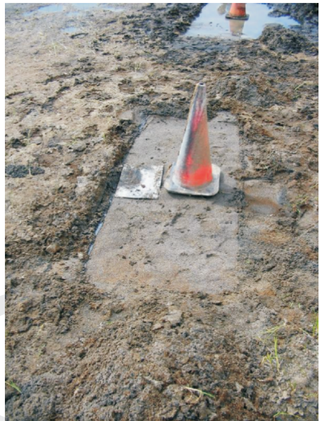
Figure 2. Orange cone and steel plate marking the location of a test coupon during excavation of 10-year samples
